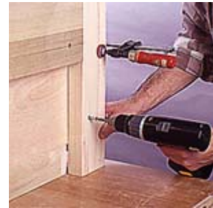
18--Position the headboard and clamp it in place. Bore and countersink pilot holes and screw the headboard to the storage box.
